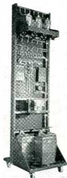
Rear view of flexible rectifier unit. Note neat appearance and ready accessibility of the parts
